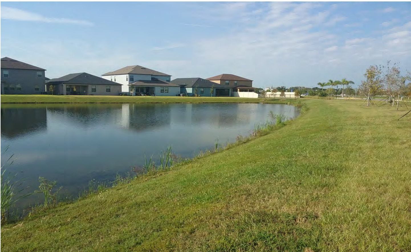
Fieldstone needs to do a better job of line trimming the bottom of the pond banks.
